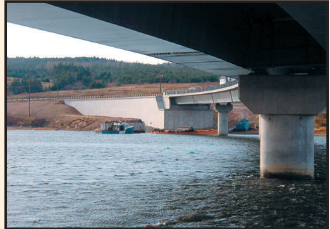
New abutments with extending retaining walls permitted keeping the same road alignment. Once traffic was diverted to the new bridge, the old bridge was demolished.
