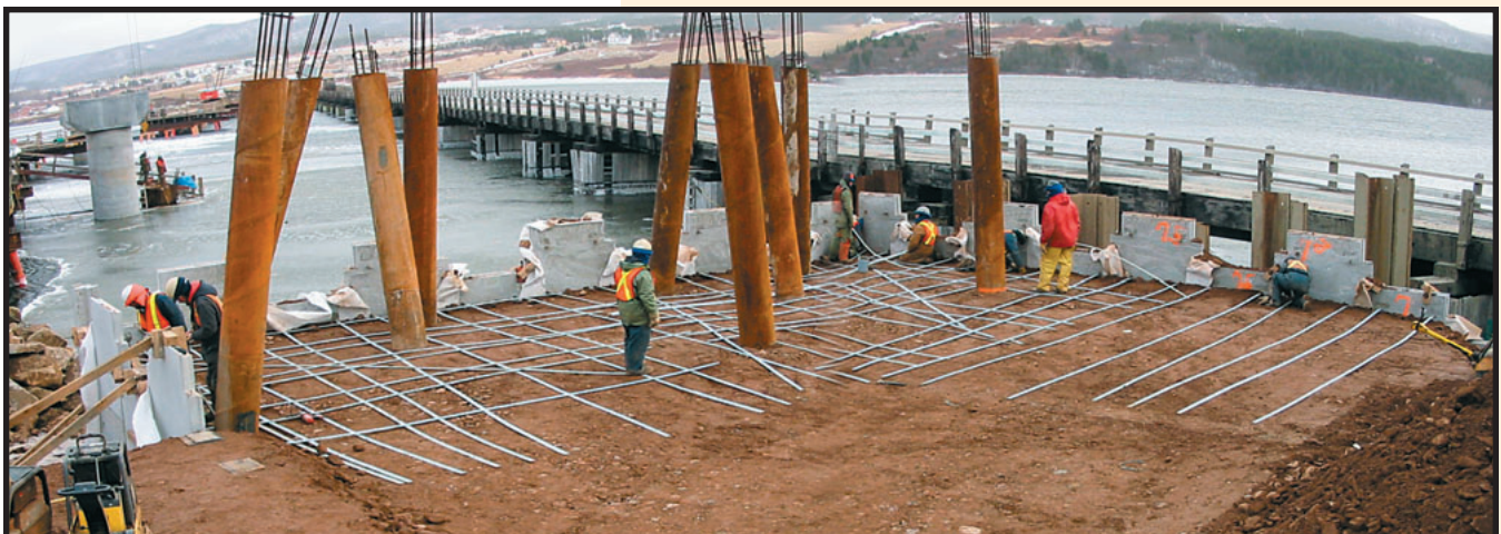
Where necessary, reinforcing strips are skewed to avoid battered piles. Note the old bridge in background.
