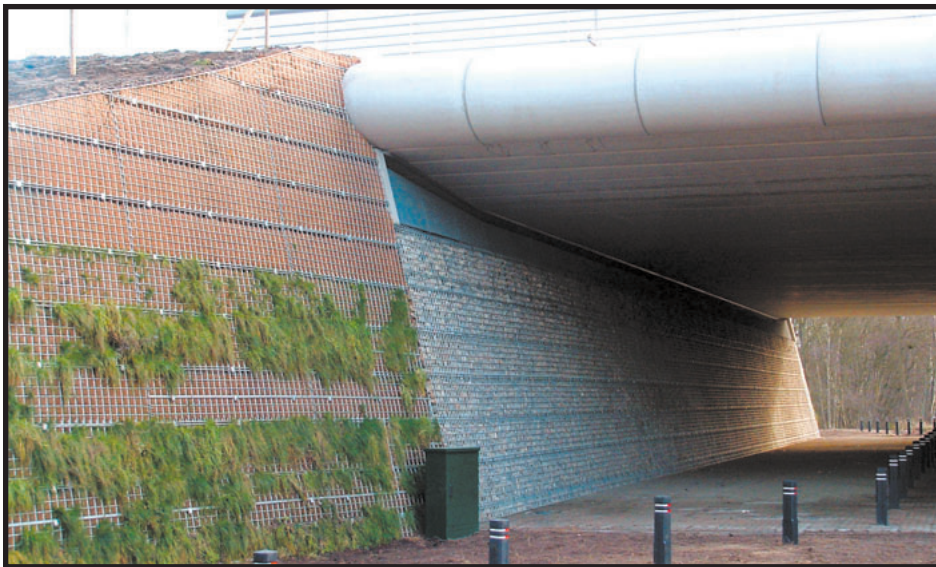
Rock faced TerraTrel abutment walls, inclined inward 15°, support the bridge structure and the high loading of the landscaping. Wing walls are also inclined and faced with organic mats that will root vegetation.
