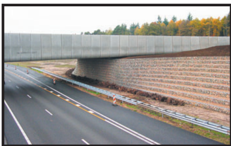
The flexibility of the TerraTrel facing is used to give the abutment and wing walls a visually pleasing contoured shape for passing motorists.
