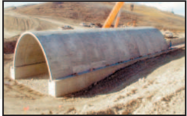
Erection of the entire TechSpan arch structure took place in two days averaging 31 lineal m (100 ft) of arch per day. Construction of the head walls and back filling followed.
